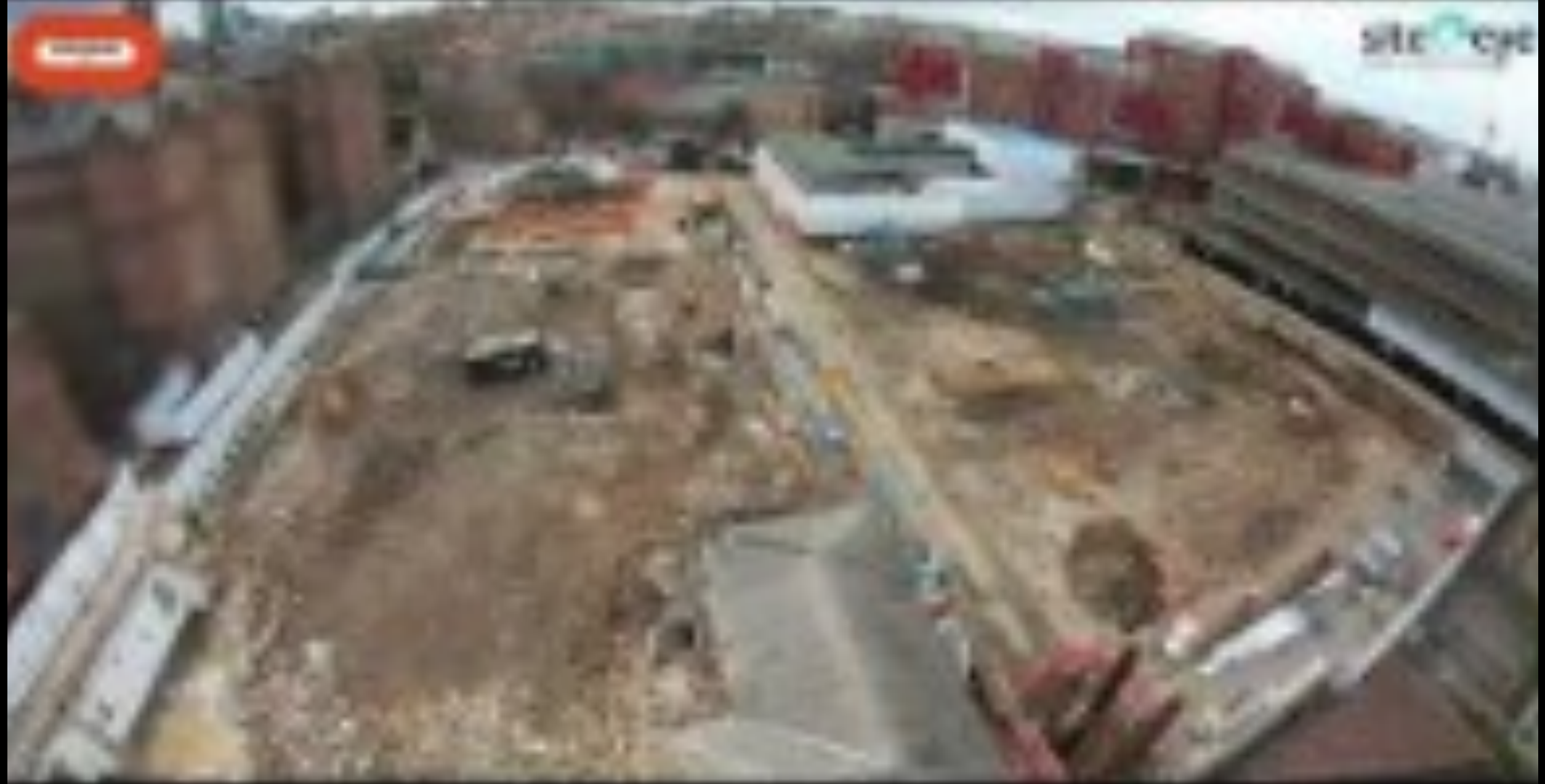
A construction method of stripping and crushing was used to reduce noise and vibration.
